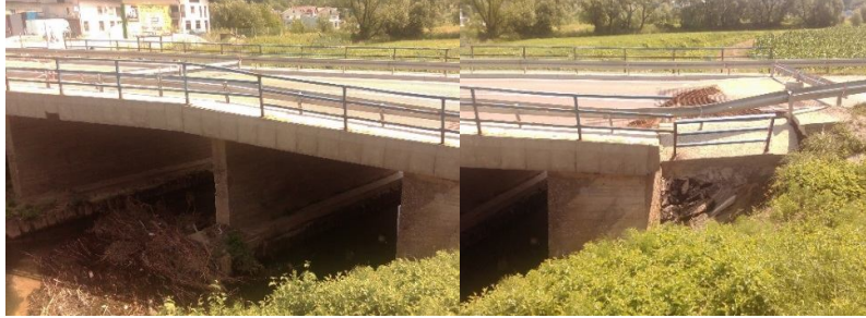
Figure 10. The Đurmanec bridge: a) accumulated floating sediment in the central opening of the bridge (left); b) erosion of the bank behind the abutment (right) / Author: M. Skazlić10
