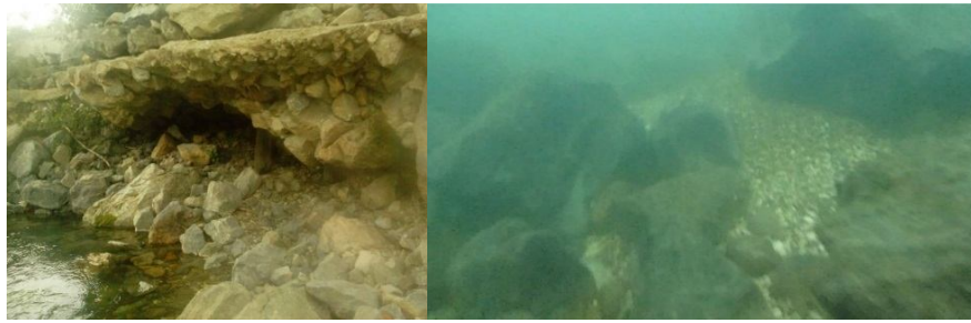
Figure 7. Detail of the collapsed rip-rap protection of piers S15: a) on the north slope (left); on the south slope (right)7
