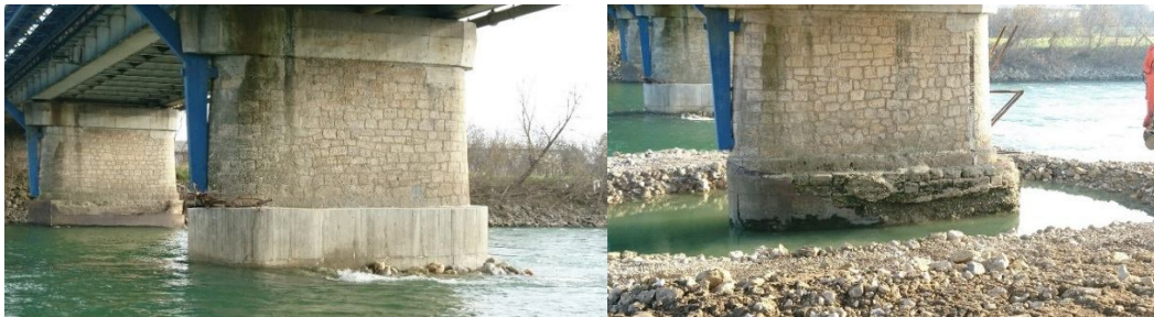
Figure 8. View from the right bank of the Podsused bridge piers: a) previously repaired middle pier (left); b) right pier during repair (right)8
