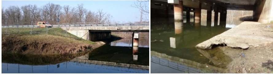
Figure 3. Collapse of the bank at the confluence of the collecting channel (left); a detail of the scoured concrete lining of the right bank (right). 3
