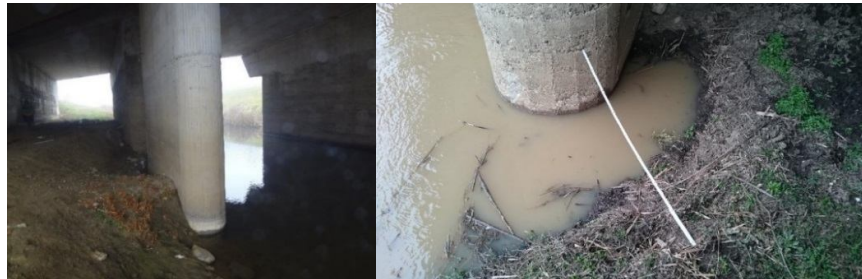
Figure 5. Erosion due to constriction of flow in the left bridge opening (left); view of the scour hole next to the upstream face of the pier S1/15
