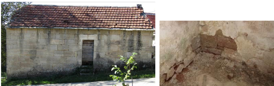
Figures 27-28. Degradation of the lower part of the northern facade (and foundation) of the house in Tomića Brig near Posušje, as a result of the capillary rise of rainwater and snow drifts, or the cycle of freezing near the ground; Due to the surface of the surrounding ground in a slope, surface water flow and flooding of the wall are present; The roof did not have a gutter, so rainwater fell from the roof onto the ground and bounced off onto the facade together with soil particles (left); detail of the interior of the house, as an illustration of the degradation (right), (photo: K. Šaravanja), [21]
