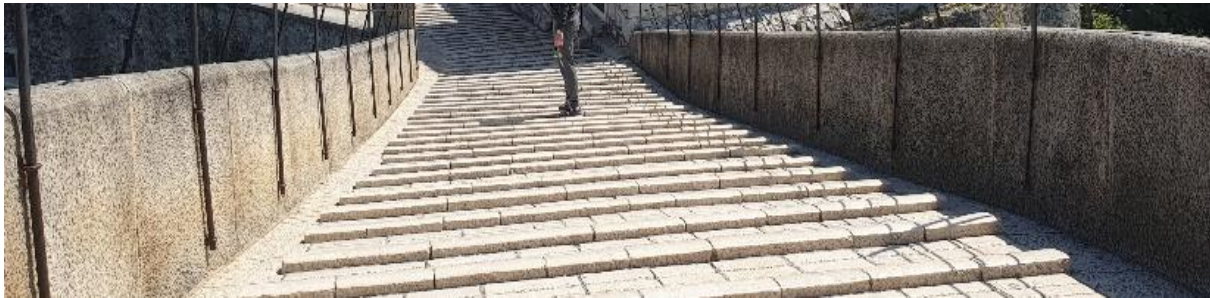
Figures 1-3. The Old Bridge in Mostar, a monument on the UNESCO list of protected world heritage: the upstream, northern side with a more pronounced patina (above, left), compared to the downstream, southern side (above, right); In addition to patina on the arch intrados, patina is visible on the parapets, cornices and vertical walls made of tenelija freshwater limestone; View from the west side of the bridge cobblestone with the inner sides of the parapet showing patina, especially the right, north side of the downstream (southern) parapet (left); damage is also visible on the joints of individual parapet blocks, and on some of them the "lime binder" is washed out, which atmospheric water has partially dissolved over a long period of time so that the joints between the blocks remain empty (below), (photo: K. Šaravanja), [21]
