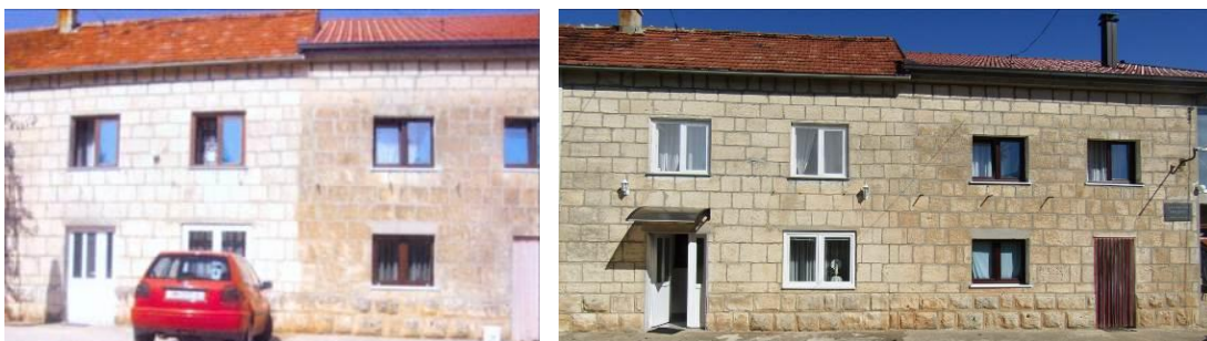
Figures 16-17. An example of removal of a layer of stone with patina from the left part of the facade made of (Posušje) miljevina on the house in Vinjani near Posušje with a special tool (pick with 3 teeth). An 8-10 mm thick layer was removed from an area of about 50 m 2 in 3 days, (left, photo: F. Oreč, 2011). Eight years later, a certain return of the patina is visible on that part of the house, (right, photo: K. Šaravanja, 2019), [21]
