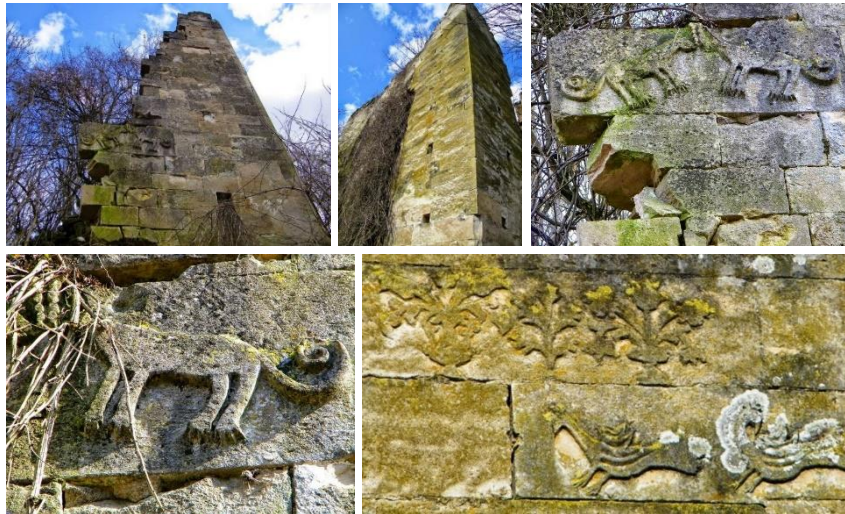
Figures 58-62. A good example of preservation of freshwater limestones miljevina in the remains of the Čengić bays' tower in the village of Rataji near Miljevina in eastern Bosnia. In addition to the patina, the presence of biological covering in the form of moss, lichens and fungi is noticeable, (photo: Zaim Bešović, 2015)
