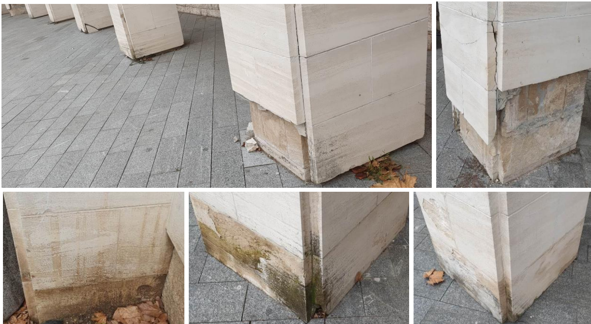
Figure 18-22. Deterioration of the lower part of the facade made of (Mostar) miljevina , which is used for decorative and protective covering in the form of a thin stone base of the Croatian Center Herceg Stjepan Kosača in Mostar due to the physical impact of atmospheric water and moisture, (photo: K. Šaravanja), [21]
