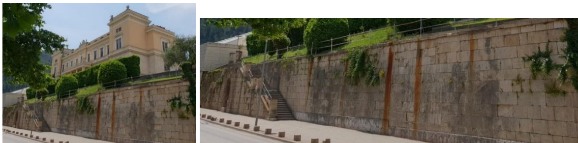
Figures 6-7. Various forms of changes to the stone in the retaining wall of the Bishop's Palace in Mostar (physical impact of atmospheric water, damage from war activities, biocolonization, damage caused by corrosion of the iron fence, anchored in the stone, which corrode in contact with moisture, and the change in volume causes cracking of stone, as well as multi-meter vertical stains on the stone, which are very difficult to remove; The stone in the building of the Bishop's Palace was repaired after the war, (photo: K. Šaravanja), [21]
