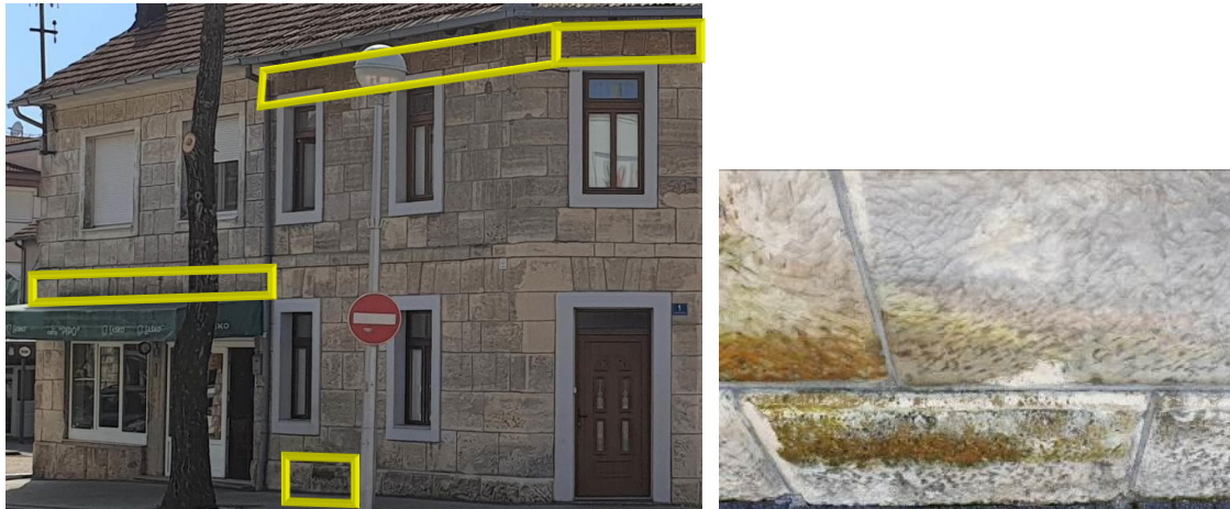
Figures 25-26. The effect of atmospheric water under the roof gutters and above the awning on a house in Posušje made of ( Posušje ) miljevina , more pronounced in the lower part of the building due to the capillary rise of rainwater (and snow), with detail (fungi and lichens), (photo: K. Šaravanja), [ 21]
