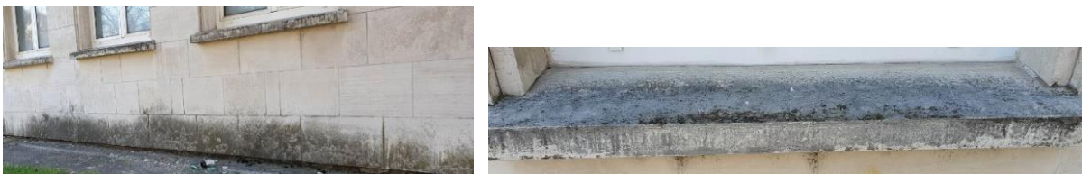
Figures 23-24. Deterioration of the lower part of the facade made of (Mostar) miljevina , which is used for decorative and protective cladding in the form of a thin stone base and stone sills under the windows of the Croatian Center Herceg Stjepan Kosača in Mostar due to the physical impact of atmospheric water and moisture, with a detail of the sill under the window, (photo: K. Šaravanja), [21]
