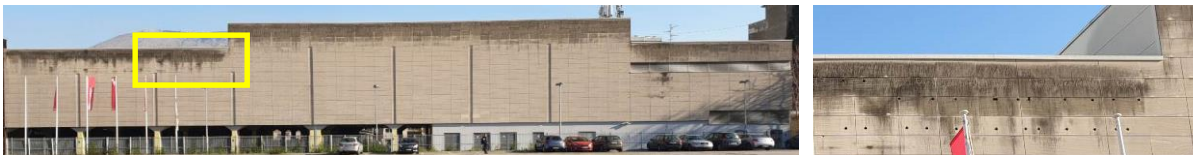
Figures 4-5. The facade of the Shopping Center "Mercator" in Mostar (left), with a detail (right), made of (Mostar) miljevina, which shows a tendency to patina the surface and a tendency to soiling when the stone is exposed to the action of seepage water from horizontal surfaces and gutters, on which there is a deposition of dust and polluting particles from the atmosphere that can stain the surface layer of vertically installed elements made of this stone, (photo: K. Šaravanja), [21]
