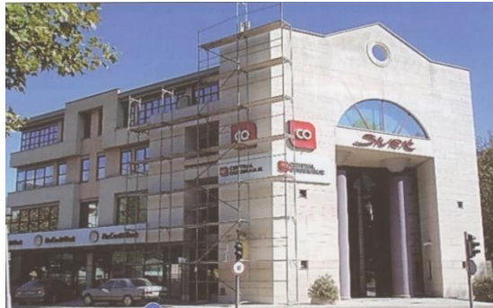
Figure 15. Removal of patina from the facade of the "Sivrića" building in Mostar made of tenelija (end of 2016), [22]
