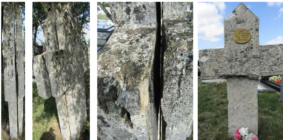
Figures 22-25. Damaged tombstones in the Radoševina cemetery near Tomislavgrad, made of stone muljika, with visible delamination along the height (figures on the left) or on part of the height of the tombstone (figure on the right) due to failure to take into account the stratification of the stone, and long-term exposure to frost, (photo: K. Šaravanja), [6]
