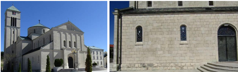
Figures 17-18. Church of St. Michael the Archangel in Tomislavgrad (above); frost-damaged blocks replaced with new cut elements of the same type of stone, (below; photo: K. Šaravanja), [6]
