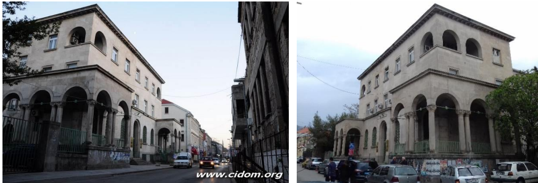
Figure 11-12. The lower part of the stone northwestern facade of the former SDK building in Mostar (left, www.cidom.org ) is more markedly covered with surface deposits of dirt than the southwestern part of the facade (right); The formation of these deposits is caused by a combination of factors related to air pollution (from traffic, heating of households and industry) and the effect of moisture on stone, (photo: K. Šaravanja), [6]
