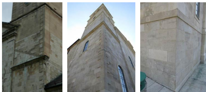
Figures 19.-21. An example of the construction of wall covering of the southern bell tower of the Church of St. Peter and Paul in Gorica in Livno with different types of dressed stone with regard to their color, size and surface processing (left), [29]; The muljika stone, which gives a special monumentality to the main facade H, it was restored on the facade and bell towers, (middle and right; photo: K. Šaravanja), [6]
